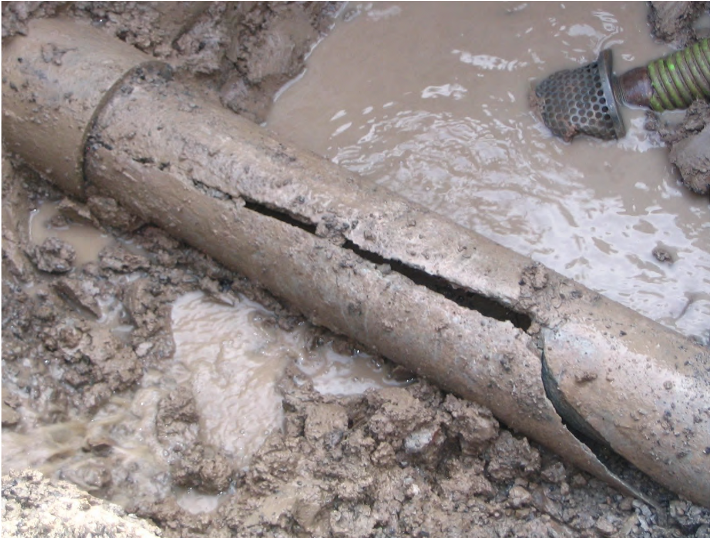
Figure 3: Longitudinal watermain break with evident Contamination.
