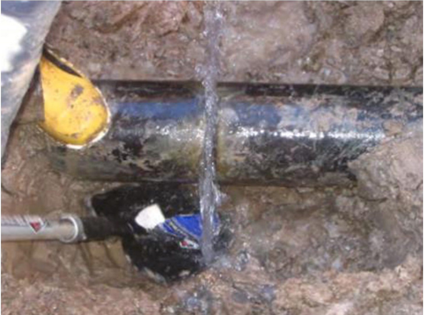
Figure 1: Circumferential watermain break with flow maintained until after an Air gap was created.
