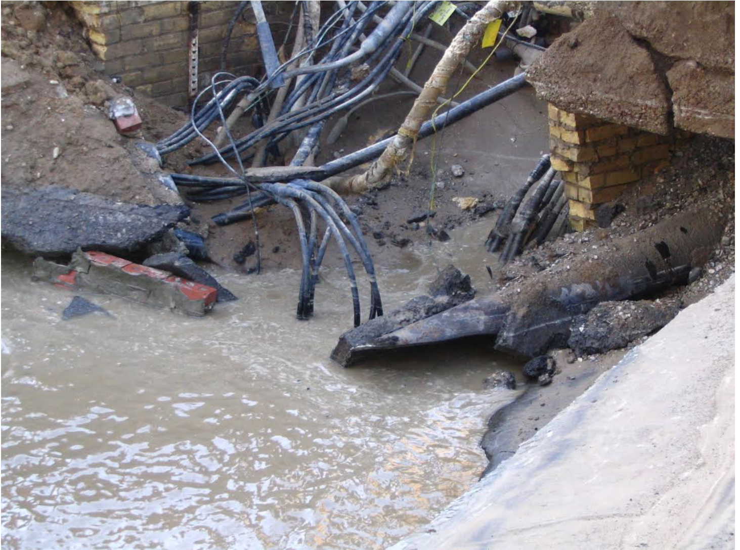
Figure 4: Spiral watermain break with evident Contamination.
