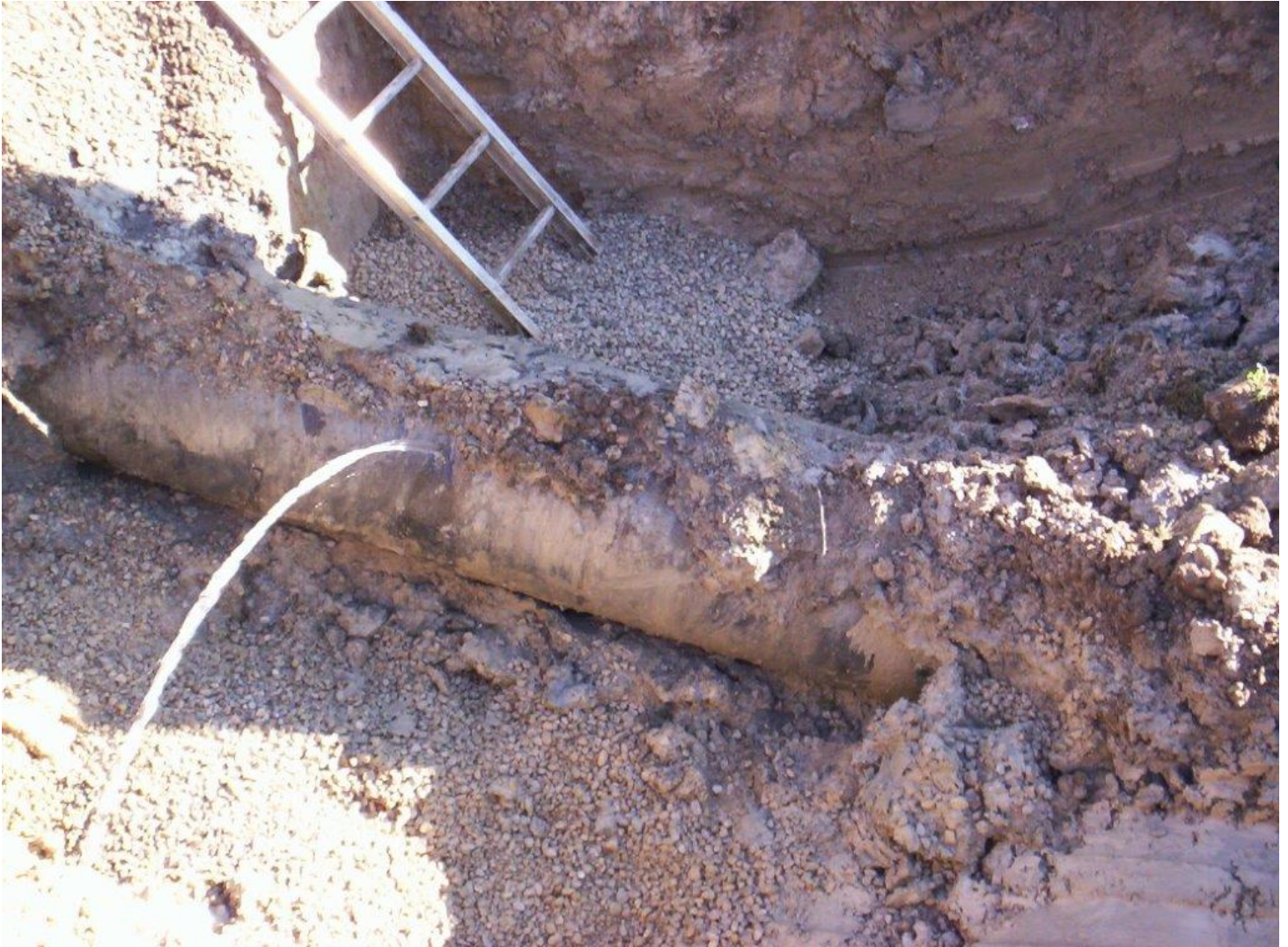
Figure 2: Corrosion hole leak in a watermain with flow maintained until after an Air gap was created.
